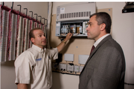
Joel Grandshaw of ComSys and Lonn McDowell of IVC in the IVC headquarters telephone room with the Toshiba Strata CIX670, which is networked to a Strata CIX100 miles away via Toshiba Strata Net networking.
